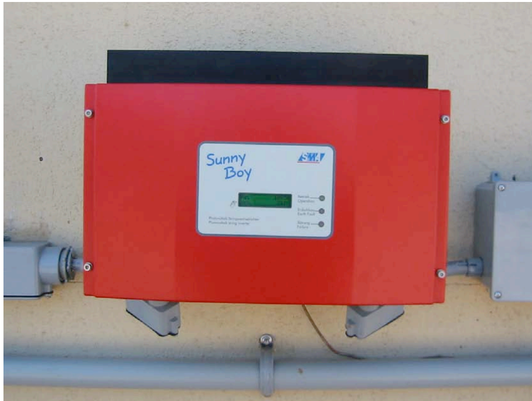
Figure 11. Utility-Interactive Inverter with Internal DC Bonding Point, GFPD, and Connection Point for Grounding Electrode Conductor
