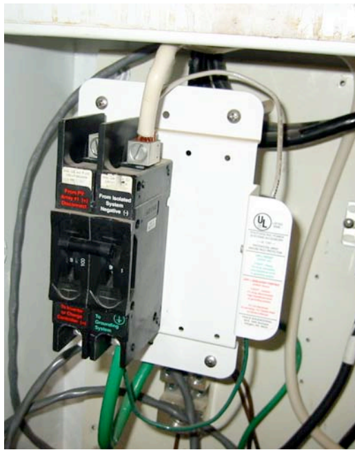
Figure 12. External Ground-Fault Protection Device
