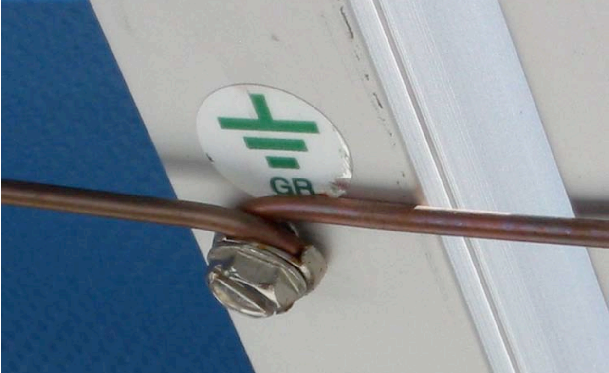
Figure G-2. Improper Module Grounding
