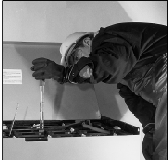
FIGURE 5.1 – Measuring specific gravity of cell electrolyte with a hydrometer
