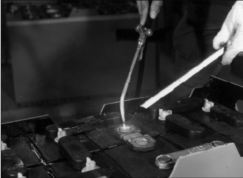
FIGURE 5.5 “Burning in” a new intercell connector to cell posts (protective cloths are removed for clarity of photograph)
